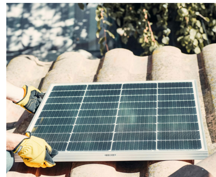
Solar Roof Top PV installations require data on the investment requirements and benefits.
